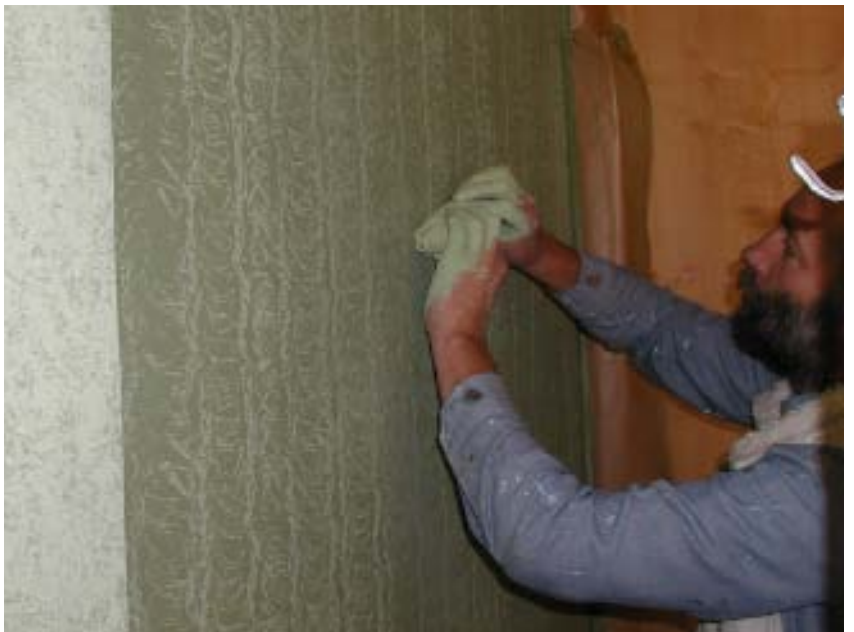
2006: the Master Painter applying the third from six paint coatings over the paper covered walls.
