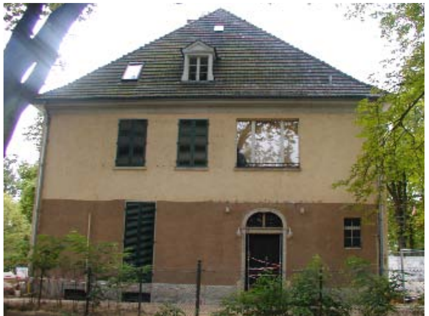
2004, beginning of the works of removal of the coatings from the last decades.
