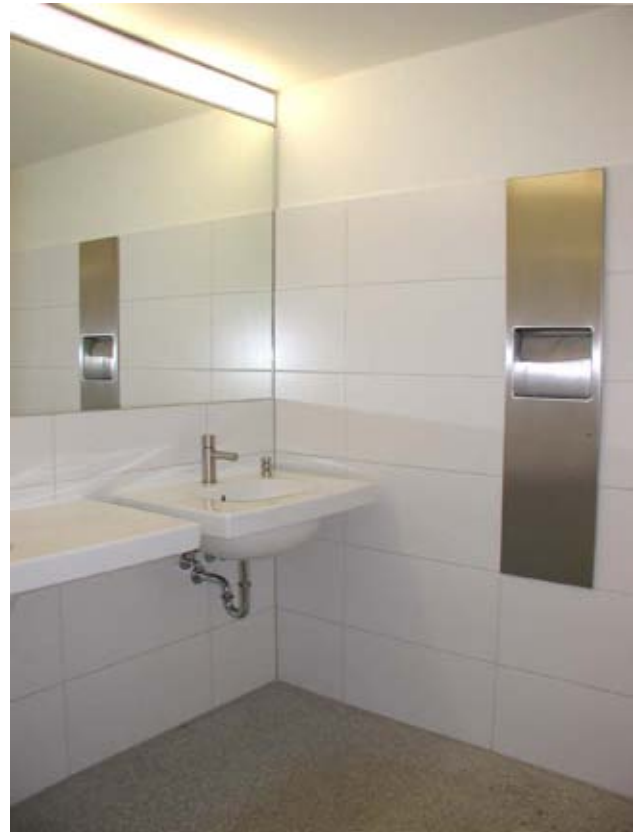
2006, washroom of the visitors' toilet area, placed in the cellar of the main House.
